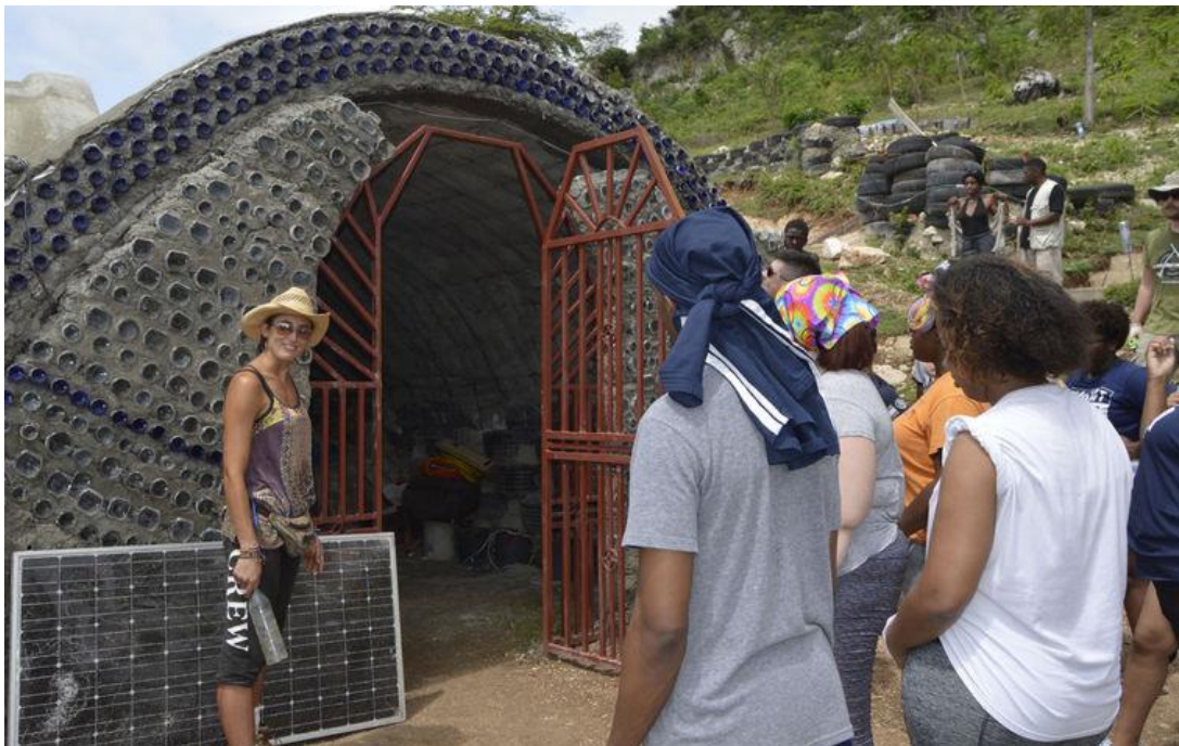
LU students help build Sakalaawel earthship project in Jacmel, Haiti. March 17, 2017. (Photo by Duwon Clark)
